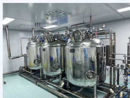
CIP/SIP Compounding System
