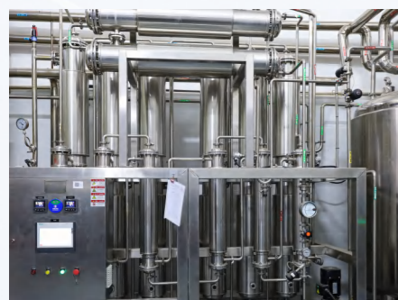
WFI Generation System
